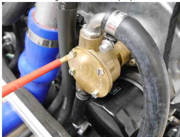
Fig. 8.13.3-3: Raw water pump
